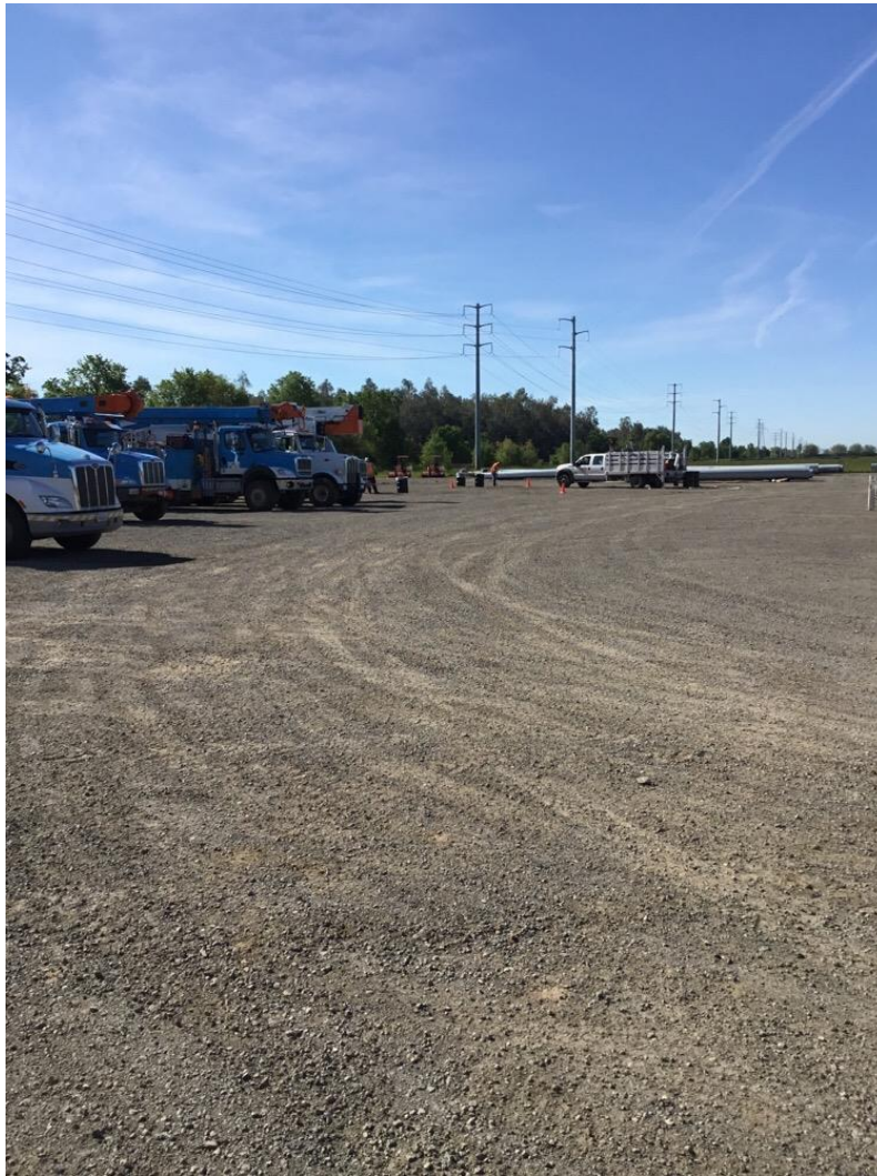
Photo 4: Crews observed cleaning up stained soil at LZ 4/31 in accordance with the project SWPPP.
